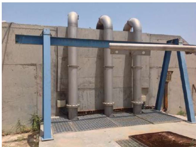
Station de relevage
